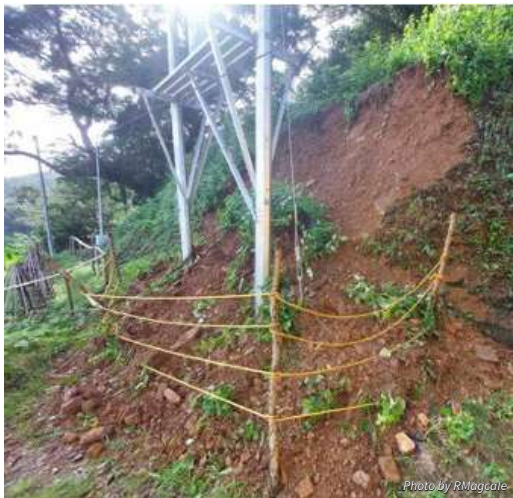
Contained loose soil around transformer area
